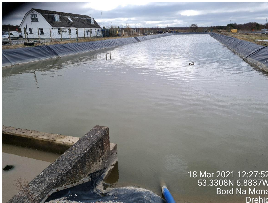
Photo 3 Lined Attenuation Lagoons South of the WMF (Wet-Well on Left)
